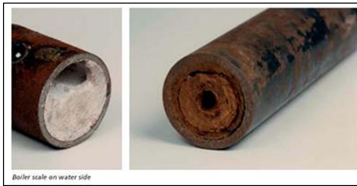
Figure 1: Scaling on pipes [2]
